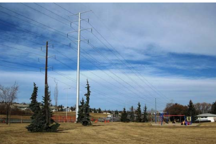
Looking north at the new Enmax transmission tower
