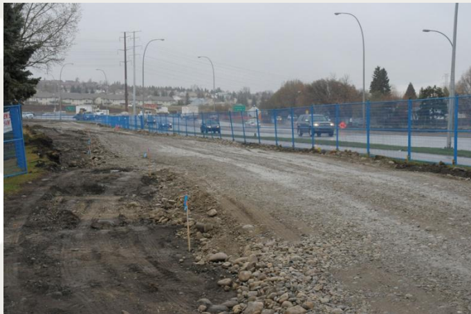
Early stages of the detour that will keep traffic flowing while the overpass is under construction
